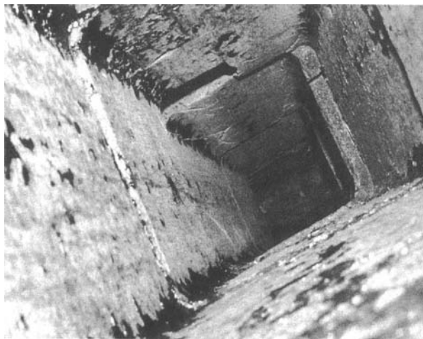
Figure 4-1. The interior of a clay flue tile-lined chimney illustrates the impact of a chimney fire – multiple cracks in tile liner sections and a missing segment of tile which fell down into the smoke chamber/damper area.
